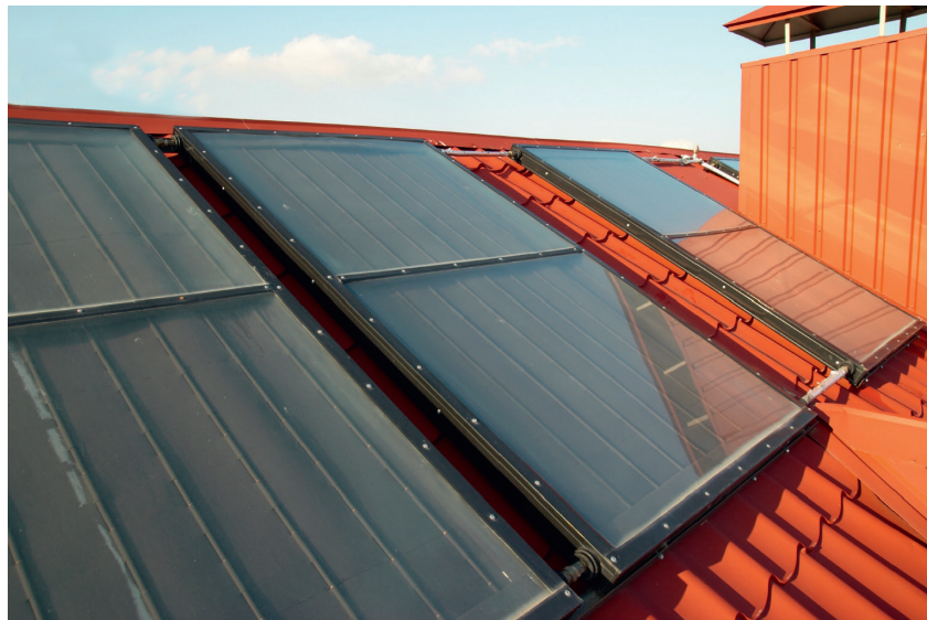
Figure 1.18 Solar hot water panel.
