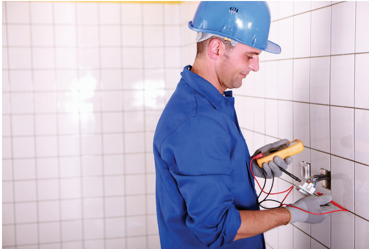
Figure 1.5 The Local Authority Building Control Body should be notified before carrying out electrical work within bathrooms.
