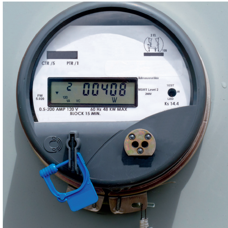
Figure 1.10 Smart electricity meter.
