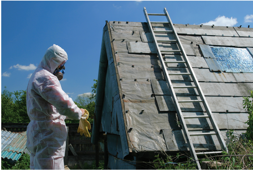
Figure 1.7 In order to work with such hazardous materials asbestos removal workers must have a licence.
