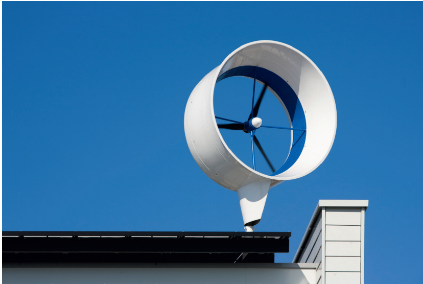
Figure 1.14 Small wind generator on a domestic property.
