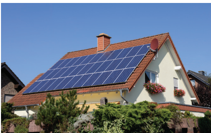
Figure 1.11 Solar photovoltaic (PV array).
